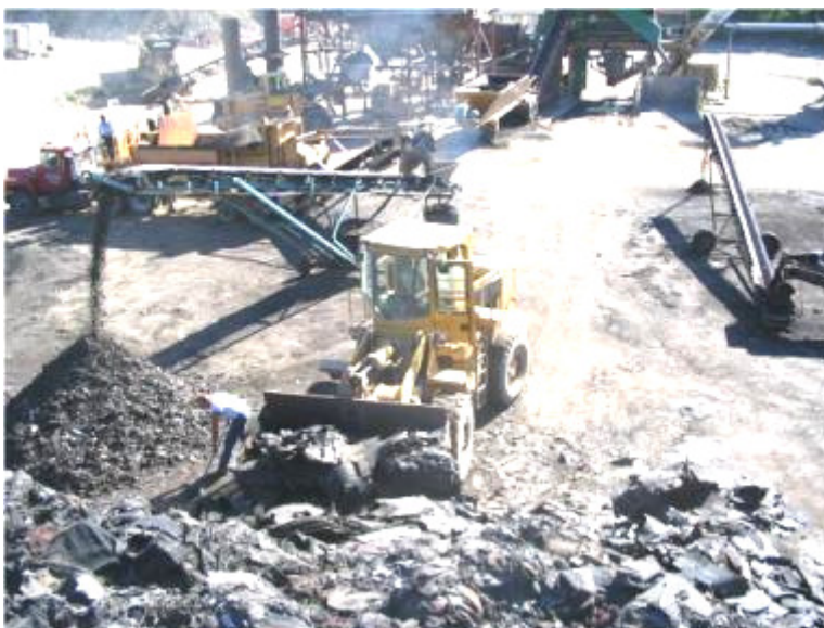
Picture 12 - Front End Loader and Operator Moving Material from a Pile of Source Separated Tear-Off Shingles
